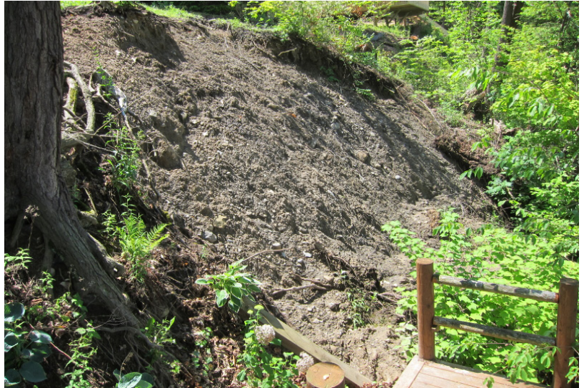
Extreme storm events coupled with poor bank stabilization and improper landscaping above the shoreline undercut the tree roots and severely eroded the bank. Soft-armoring may still be an option to restablize this slope. Photo by John Sutton.
